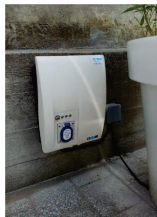
Home installation – France
