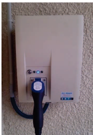
Home installation – France
